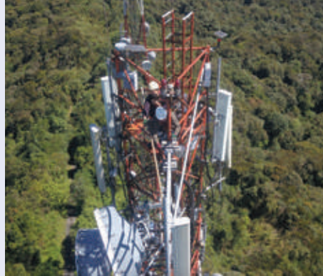
Tower with Greenhouse Gas Monitoring System
